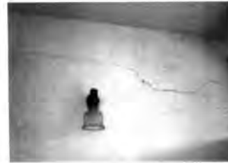
Figure 6: Horizontal cracking under beams
