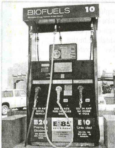
Fig 1. Biofuel pumping station
